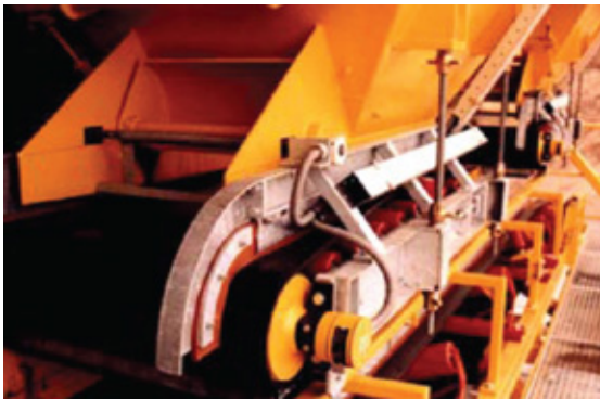
RULMECA 8.5" Dia 4 HP Motorized Pulley at 200 FPM driving a 30" W feeder belt on 1 of 2 hopper feeder conveyors beneath aggregate mixing bins at a Cement Plant.
