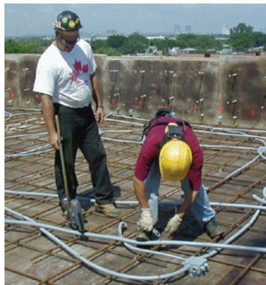
Figure 21: Tying electrical conduit using the rebar tying machine (left) and manual tying with pliers (right).
