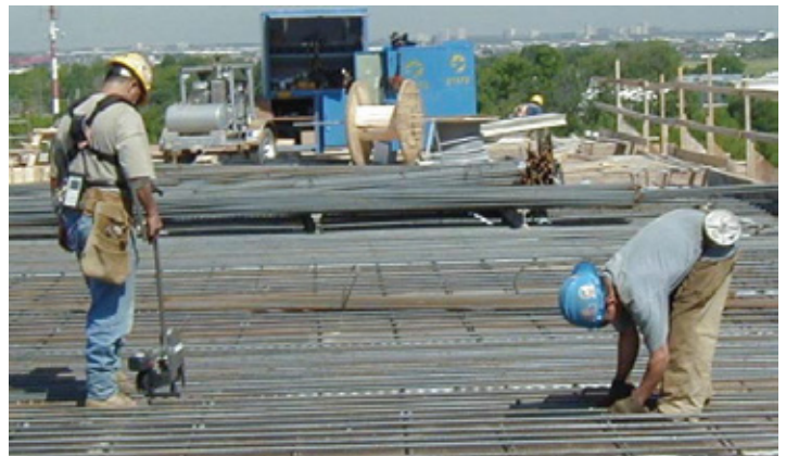
Figure 4: Rebar tying using a rebar tying machine (left) and manual tying using pliers (right). Dababneh and Waters (2000) reviewed the literature on the ergonomics issue of rebar tying, and concluded that properly designed powered tying tools may be the best ergonomic solution. Extended tool-body design or extended arm attachments can be used to eliminate the need for stooping when working on a horizontal platform (see Figure 6). Also, tools with a pistol grip would allow workers to tie horizontal or vertical rebar while keeping their wrist straight and reducing the need to perform high twisting or bending motion of the wrists (Vi, 2003).
